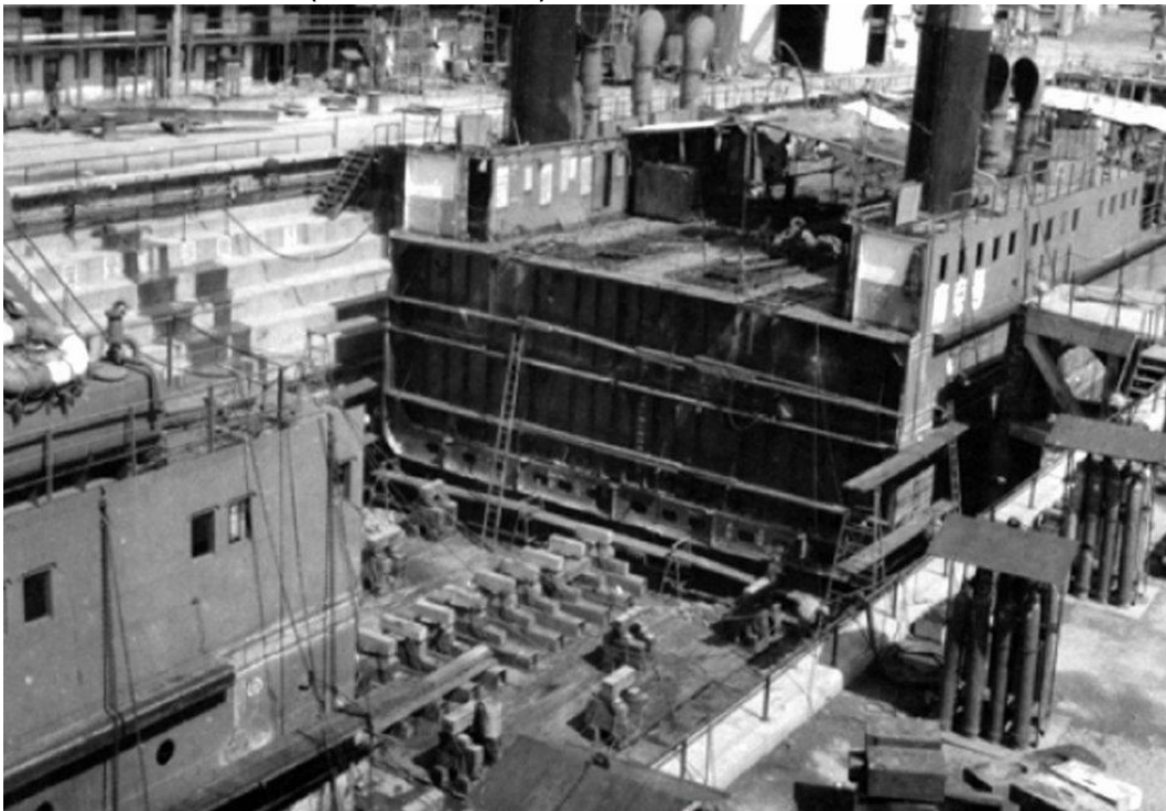
Being repaired in 1955 at Shanghai Shipyard after being raised in two sections (Internet).
